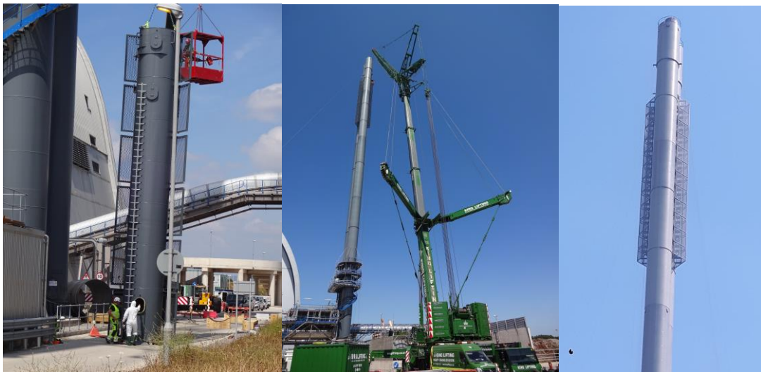
Dampers and side panels at ground level
